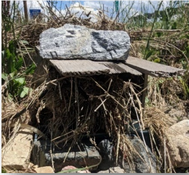
Figure 14. Ditch flume stuffed with vegetative debris after a storm event on July 1, 2021.
