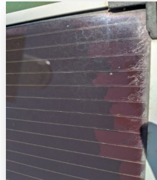
Figure 22. Deteriorated solar panel at the MFD site.
