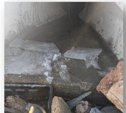
Figure 15. Broken up ice sheet inside the culvert at the MFD site during the winter months.
